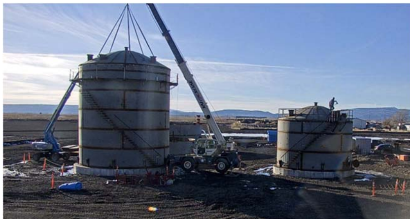
Construction progress, Red Rock Biofuels Lakeview facility. (Source: 2019 DOE BETO Project Peer Review Update 5 March 2019)
